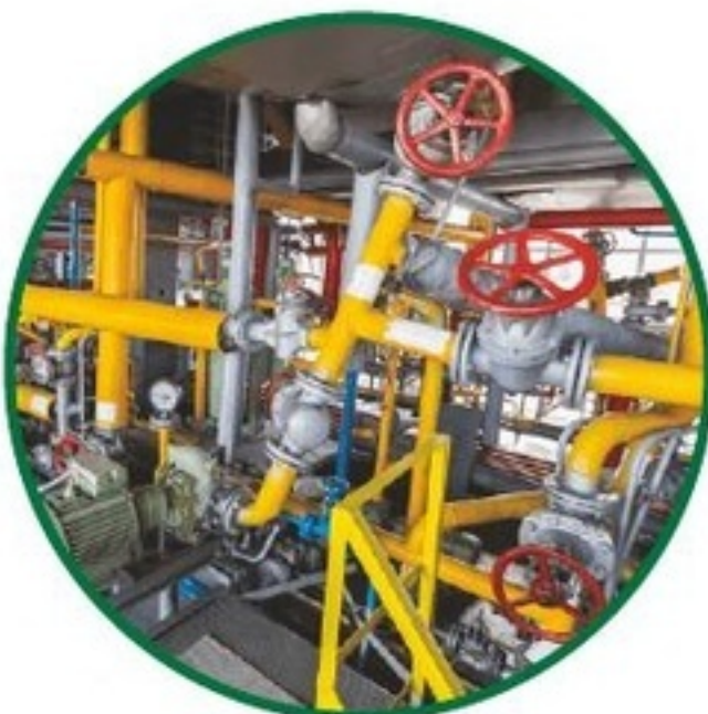
Fat Modification Plant
