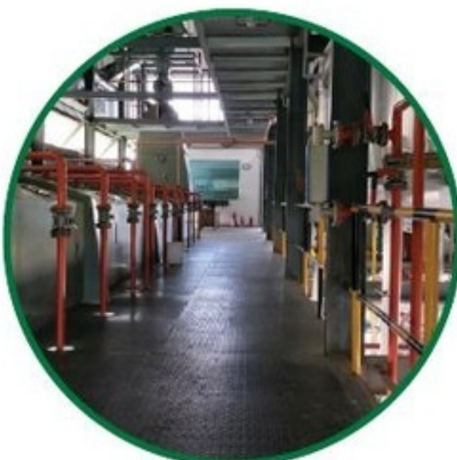
Solvent Extraction Plant
