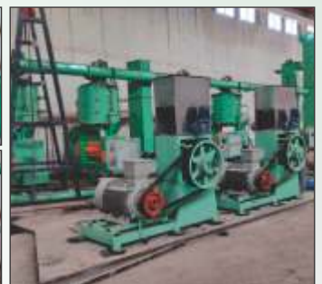
Installed in India
