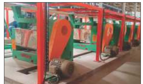
Installed in India
