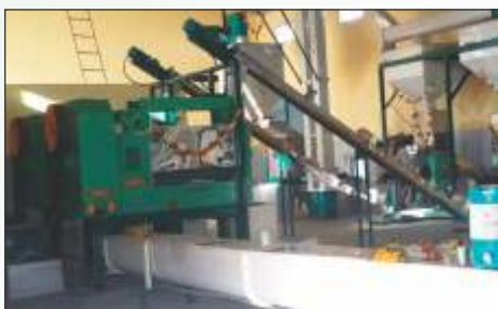
Installed in Nigeria
