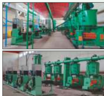
Installed in Nigeria
