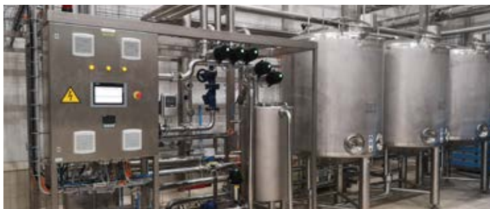
CIP (Clean In Place) units
