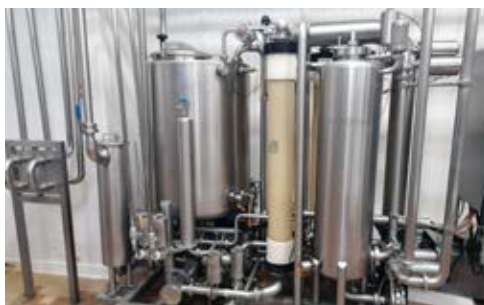
MF - brine microfiltration Units
