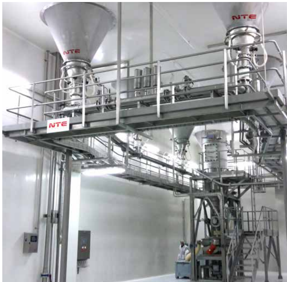
Complete system for Storage, Dosing, Material Handling and Packing
