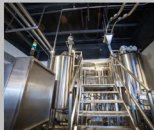
Brewing block for manual operation (5 hl, 10 hl and 17 hl)
